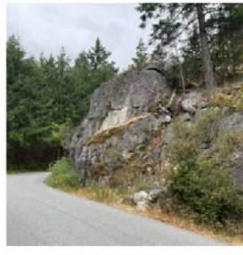
2 Rock scarps. Evidence of significant potential for a future rock slide.
