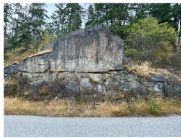
3 Rock scarps. Evidence of significant potential for a future rock slide. Joints present (Marked pink on the previous plan provided by GES, June 24, 2022)
