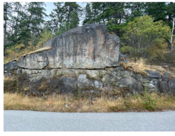
3 Rock scarps. Evidence of significant potential for a future rock slide. Joints present (Marked pink on the previous plan provided by GES, June 24, 2022)
