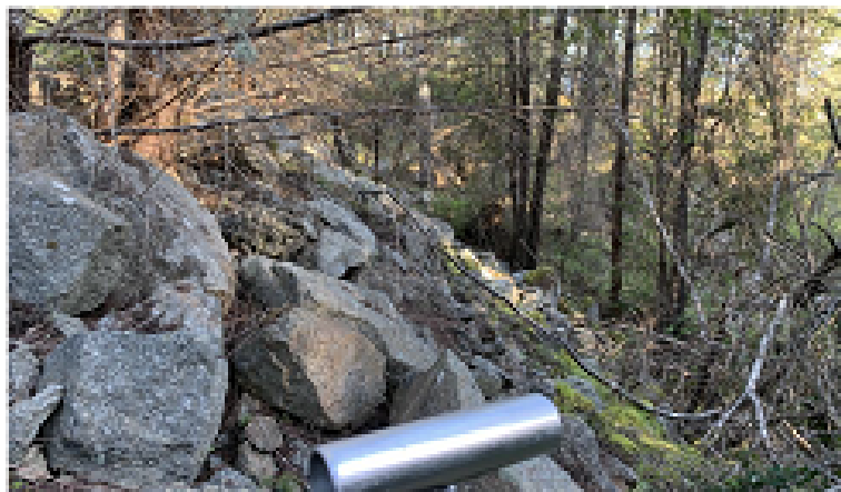
Photo 2: Loose Surface Rock Blocks Zone ("Zone 2")
