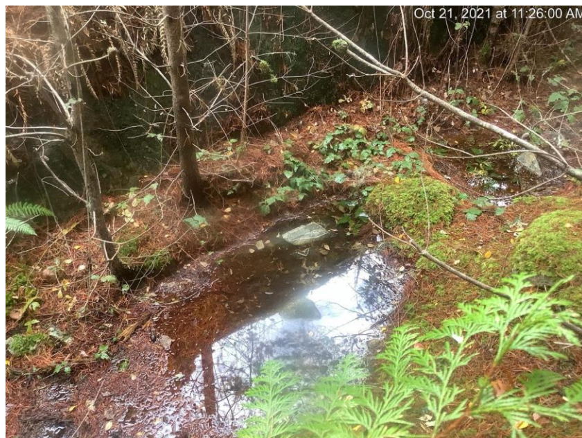
Photo 11. Pooled water in ground depression beside unfinished road in middle of property
