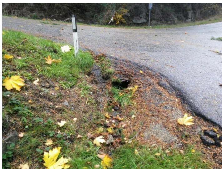
Photo 2. Existing stormwater control requires assessment
